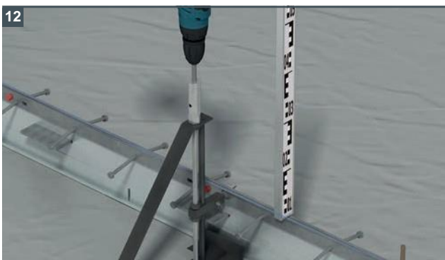
12 Check the height and adjust where necessary using the nut on the jack.
