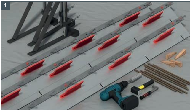
1 Set up the site. Laser dumpy level set up, finished floor level datum taken, membrane laid, hand tools available
