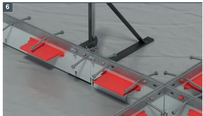
6 Continue to fit the ArmourJoints. Ensure the lapped joints are butted end to end tightly. Fit the plastic bolt and wing nut at the lapped joint.
